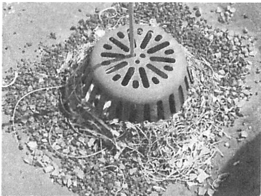
Photo #3: Debris along drain on the newer sections
